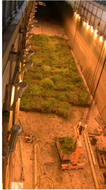
Figure 3.1 Upper panel: Experimental test-section in the Large Wave Flume (Grosser Wellenkanal, GWK) (from Möller et al., 2014). Lower panel: view of the vegetated test section at the mid-point in construction, looking towards the wave paddle (photo: I Möller)
