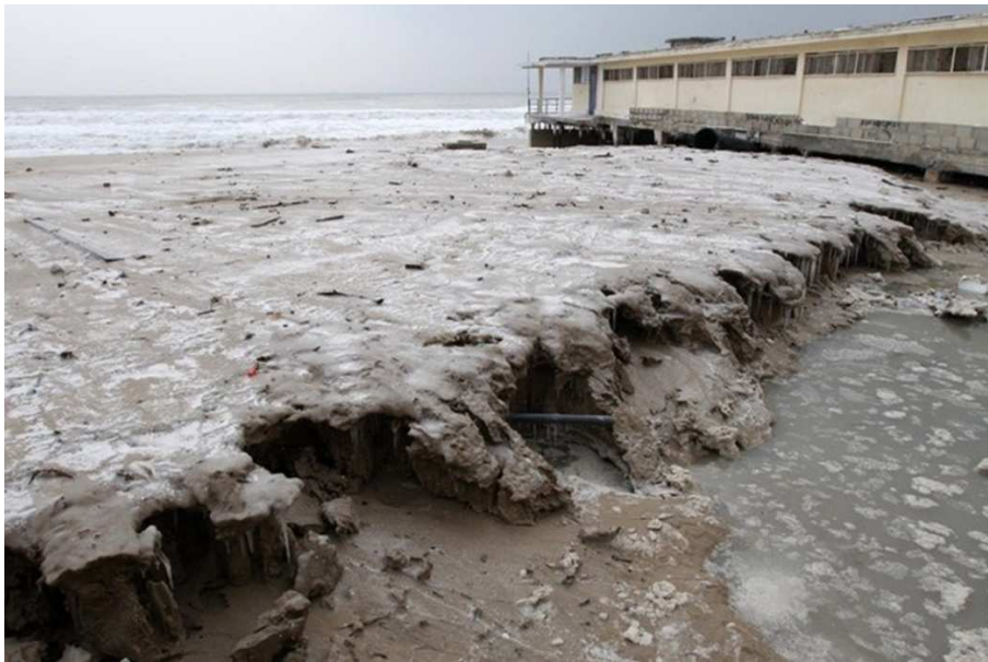
Figure 2.9 Flooding of Varna Central beach (north), undermining of Sea Baths foundation, damages to the buildings and beach erosion (Source: dariknews.bg).
